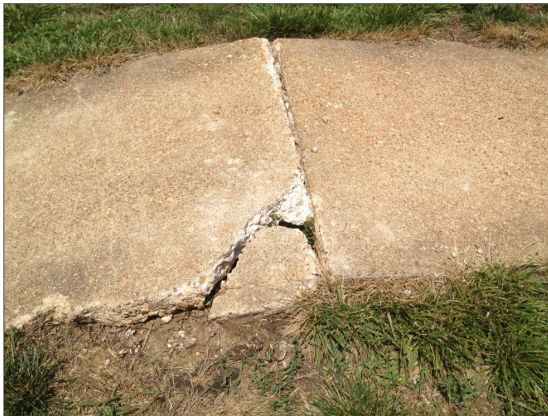
Figure 20. Broken and Uneven Sidewalk Segments
