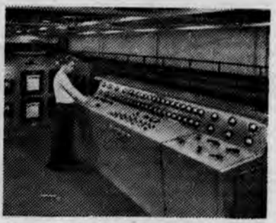
Console of controls for entire process is readily operated when necessary, even though seldom used in the almost fully automatic operation.
