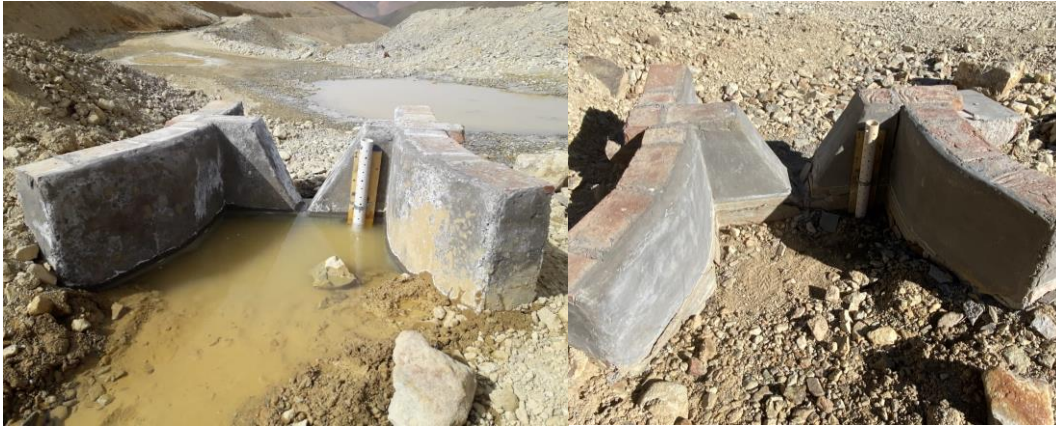
Figure 3.3: V-notch weir at the outlet of Altar watershed. After construction (left side) and after a year (right side). (W1, Figure 3.1). Notable erosion after a year is observed on the v-notch.
