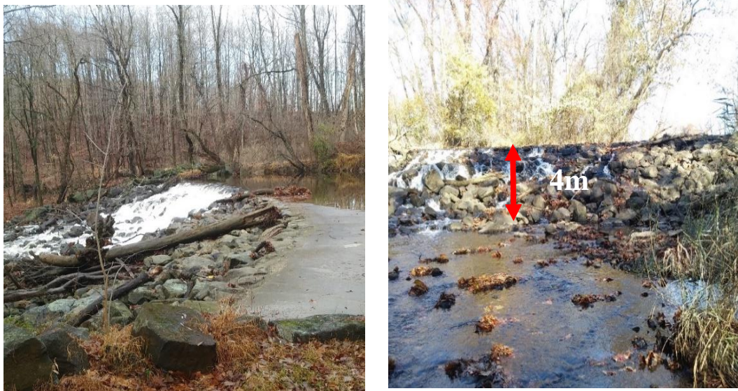
Figure 3.2: Images of water and large debris flowing over Cooch's Mill dam (left) and view of downstream of dam (right).
