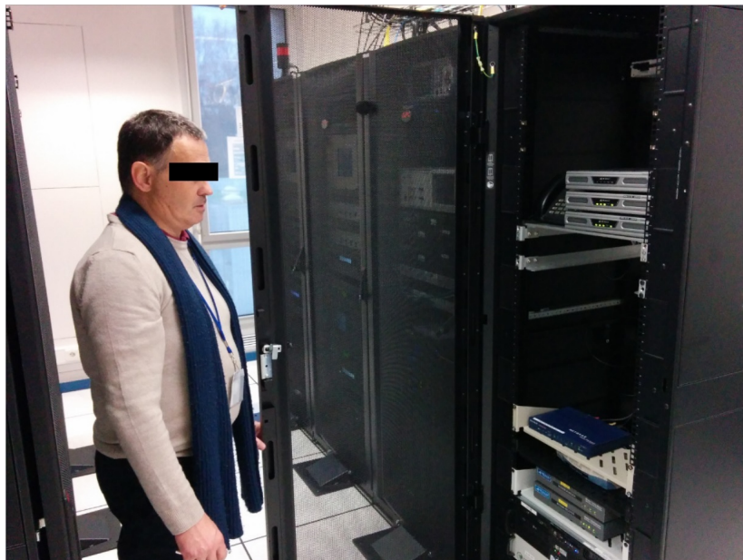
Figure 2.26: Satellite Terminals in CNES
