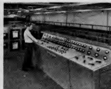
Console of controls for entire process is readily operated when necessary, even though seldom used in the almost fully automatic operation.
