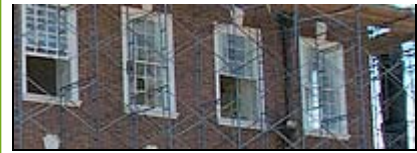
A member of the construction crew works on the exterior of Wolf during Phase II
