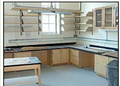
The future third floor Biodiversity Laboratory towards the end of Phase III construction
