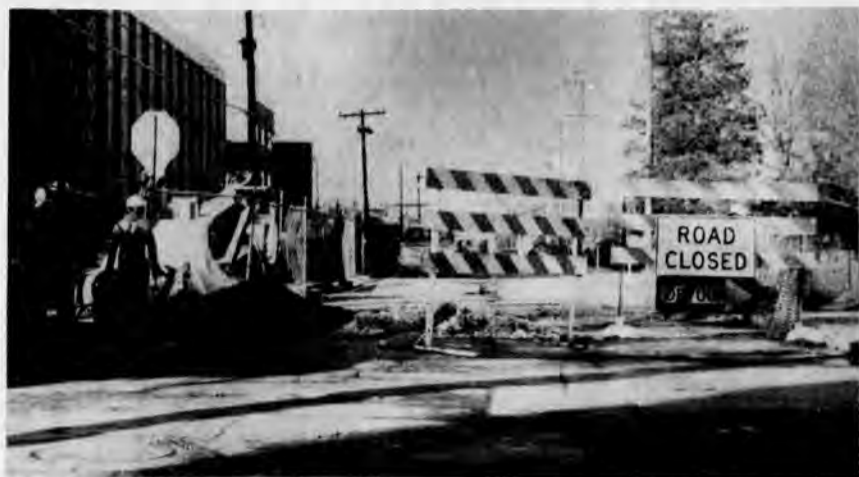
Traffic was blocked on Academy Street last week while electrical conduits and sewer lines were installed for the improvement of Colburn Laboratory.
