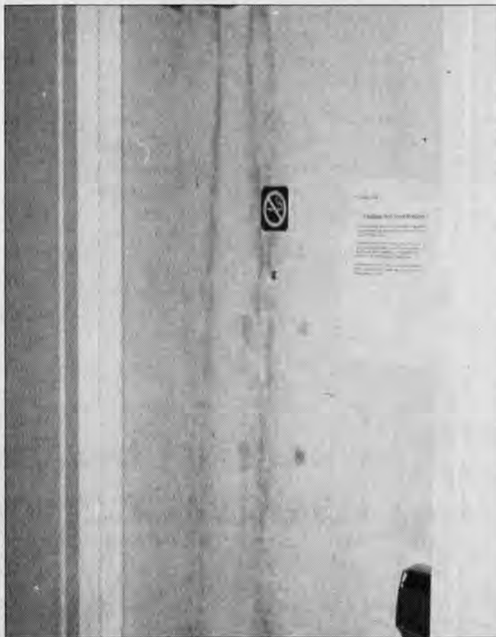
THE REVIEW/Erin Klein The door of 1509 Christiana West Tower was coated in soot Friday afternoon following a kitchen fire.
