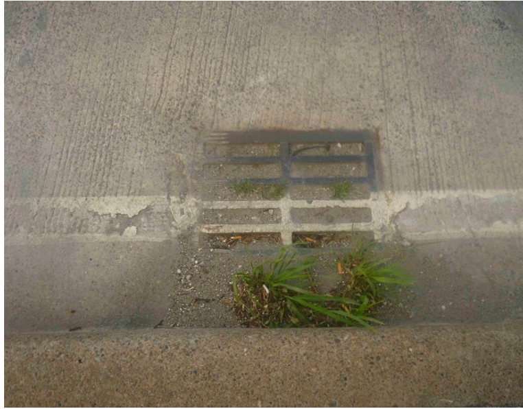
Figure 2.16: Example of blocked scupper.
