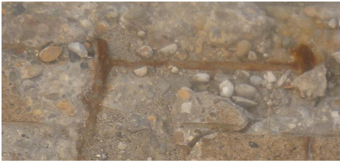
Figure 2.6: Corrosion of reinforcing steel.
