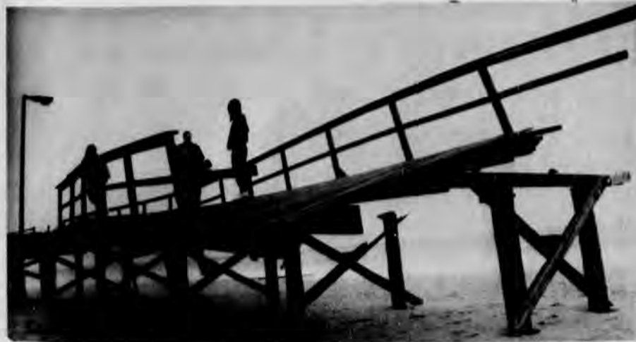
Damage to Dewey Beach from the January 1992 storm which ravaged Delaware's coastline will finally be repaired this summer with the aid from the beach restoration project.
