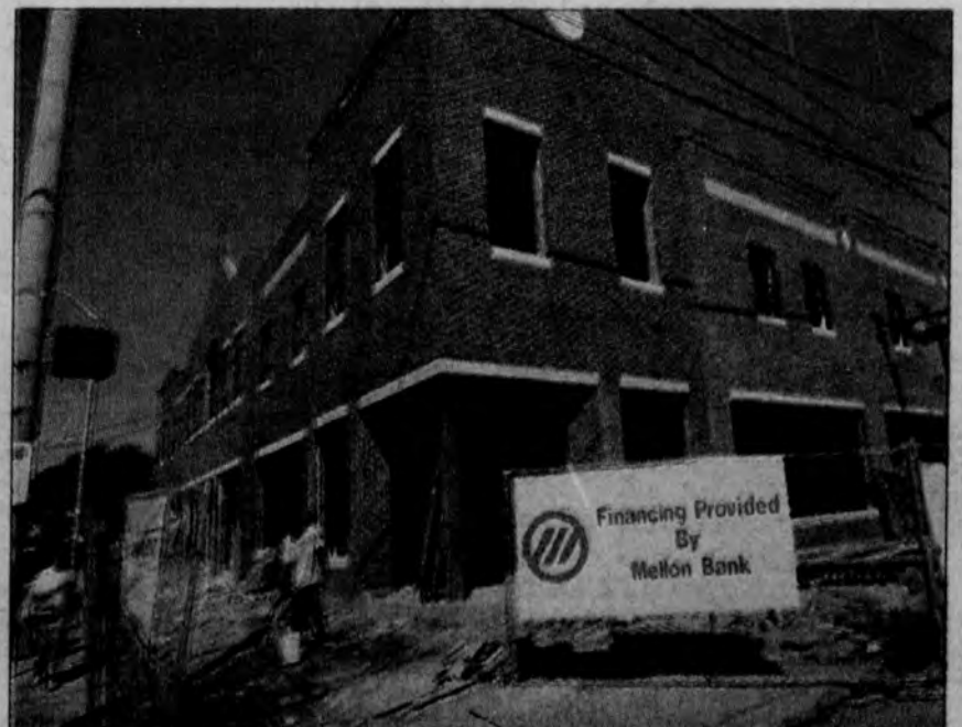
Astra Plaza Main Street, under construction at the corner of North Chapel and Main Streets, is expected to open as early as Sept. 1.
