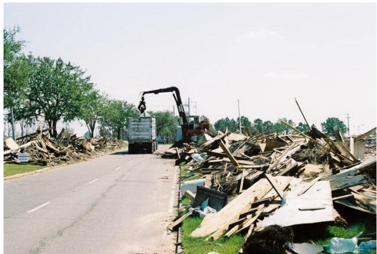
Slidell, Louisiana (September 2005) — Construction Crews begin removing debris from the devastated area.
