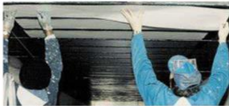
Attaching composite laminates to the underside of a bridge's floor beams. (Photograph courtesy of Dr. Michael Chajes)
