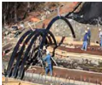
Figure 2. FRP Arches being lowered into place. Photo 6. FRP Arches being lowered into place. Reprinted from Project case studies for IBRC and IBRD Programs , D. Paterson et al., 2012, FHWA report, p.860. Unpublished internal document of FHWA.
