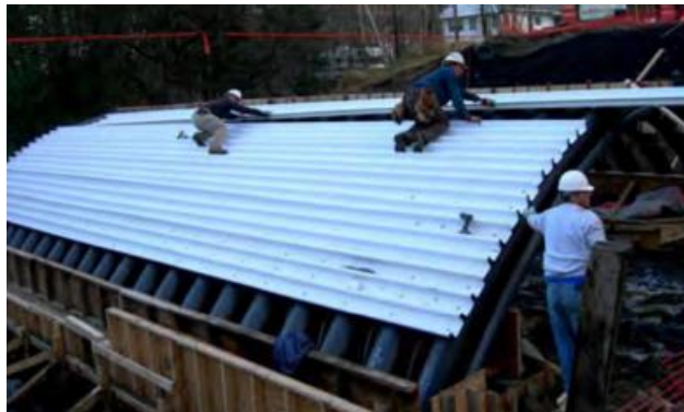
Figure 3. Sheet metal installed on FRP tubes. Photo 7. Final arch placement with corrosion resistant decking being installed. Reprinted from Project case studies for IBRC and IBRD Programs , D. Paterson et al., 2012, FHWA report, p.861. Unpublished internal document of FHWA.
