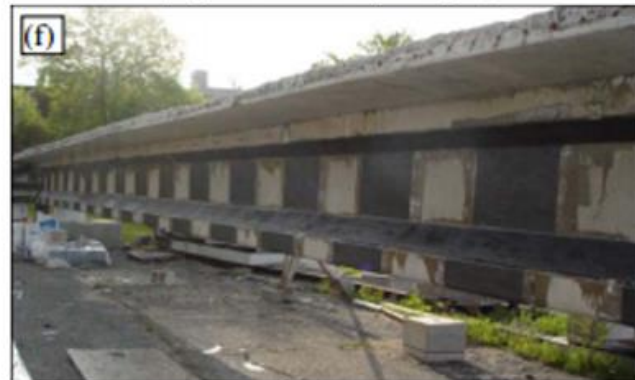
Final rehabilitated pre-stressed concrete girder with vertical CFRP strips and anchoring longitudinal CFRP strips (Figure from Cerullo, et al. (2013). With permission from ASCE. This material may be downloaded for personal use only. Any other use requires prior permission of the American Society of Civil Engineers.)
