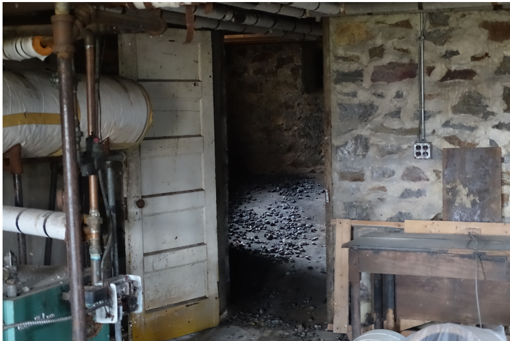
Figure 34 The basement of the abandoned cottage at Winterthur: pieces of coal litter the ground around the building's furnace. Photo by Natalie Wright.
