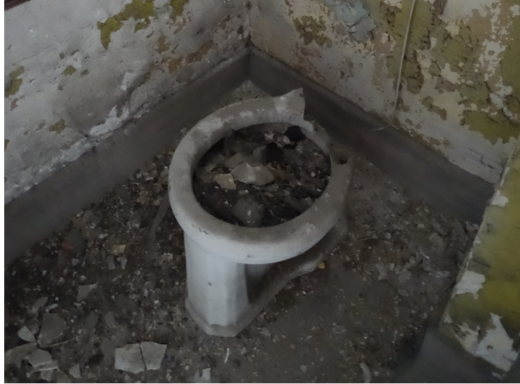
Figure 31 Broken things: a smashed toilet seat. Photo taken by Natalie Wright.
