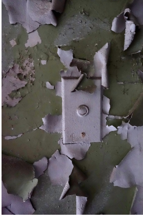
Figure 24 Detail of peeling paint. Photo by Natalie Wright.
