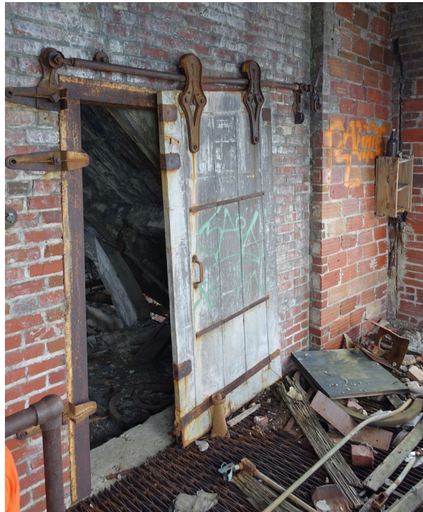
Figure 21 The sliding door in the elevator operating room at the abandoned bank. Photo by Natalie Wright.
