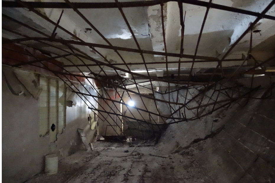
Figure 33 An otherworldly scene: a ceiling has fallen down to reveal its structure beneath. Photo by Natalie Wright.
