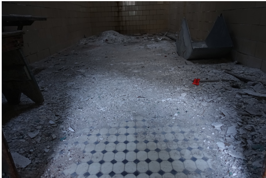
Figure 87 A bathroom floor peeks through dust and debris. Photo by Natalie Wright. Eastern State Penitentiary, Philadelphia, PA.
