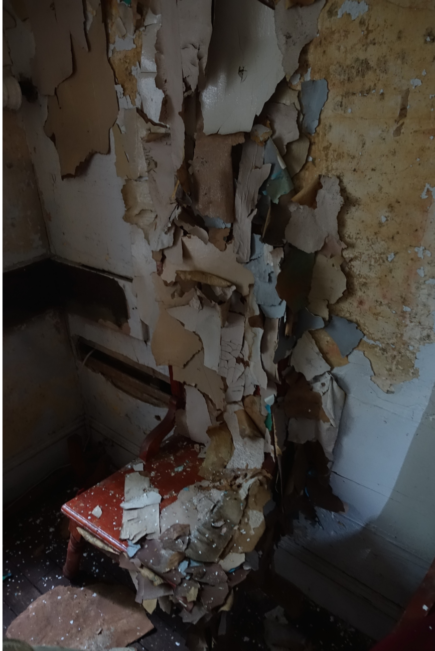
Figure 112 A tall gothic revival chair is engulfed in peeling paint and debris in Philadelphia's abandoned Hawthorne Hall. Photo by Natalie Wright.
