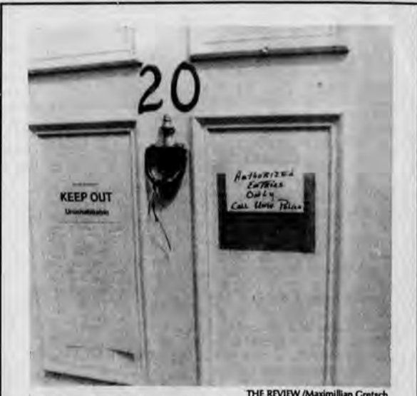
THE REVIEW/Maximilian Gretsch The front door of Sigma Nu's fraternity house bears signs forbidding entry because fire codes violations.
