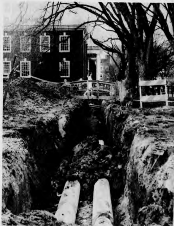
A student crosses temporary bridge, near Sharp Lab, over the construction of the university's new water recycling system.
