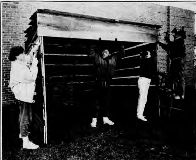
Workers (from left) Jen Chastain, Guy Wellman, Stacy Slone and Julie Wellman finish constructing manger at Ebenezer.
