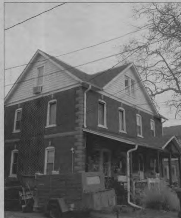
Window openings were boarded up as a fire heavily damaged the second floor of a duplex on Prospect Avenue in Newark.
