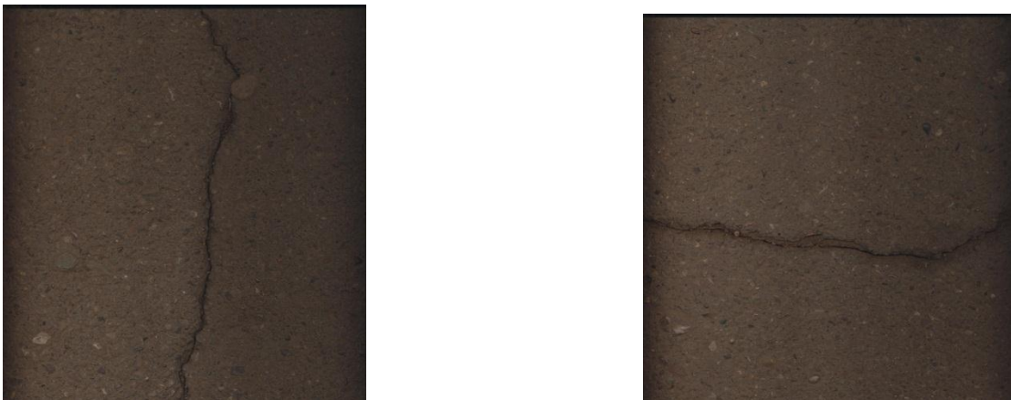
Figure 13: Original longitudinal and transverse cracks (Nejad et al 2011)
